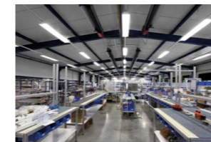
1 st lighting scene:
